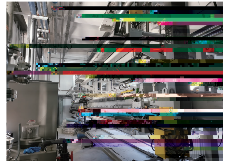
Wastewater Treatment Station
